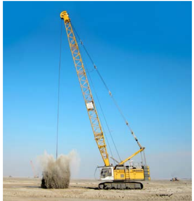
Dynamic soil compaction with a HS 8100 HD in the desert in Kuwait
