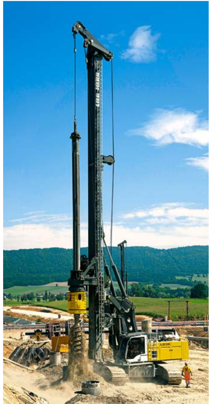
The Liebherr rotary drilling rig LB 36 operating on a construction site in Switzerland
