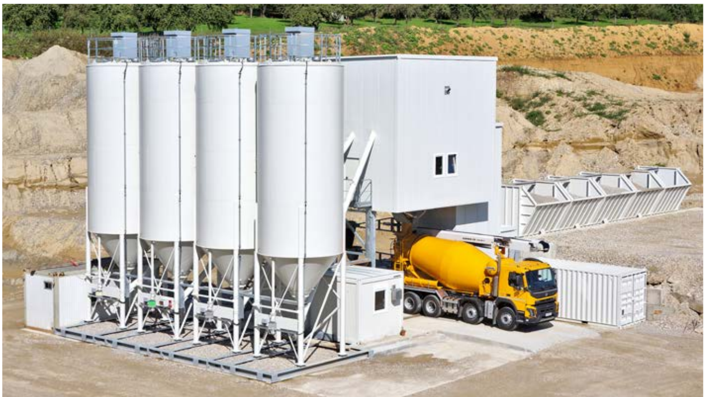
At Kohler & Müller in Engen-Welschingen (Germany), the concrete mixing plant, type Betomix 3.0, produces up to 110 m 3 of concrete per hour
