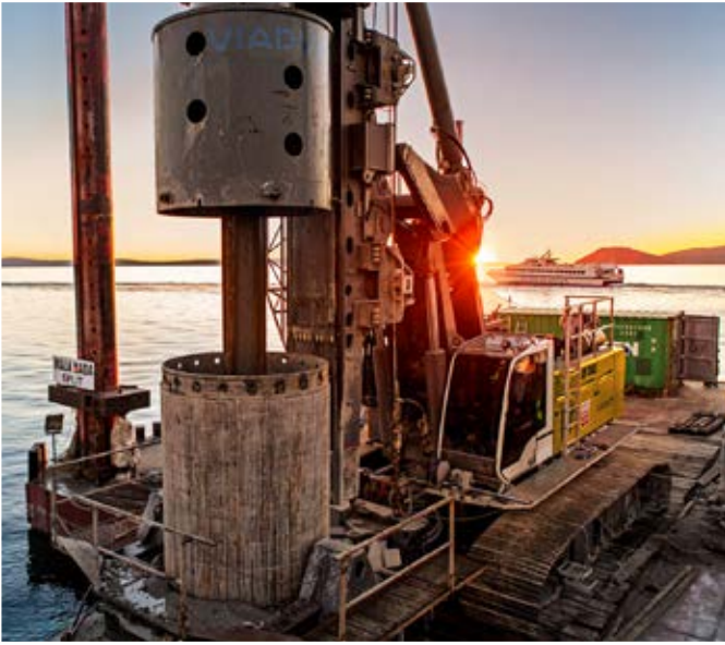
A Liebherr rotary drilling rig during drilling operations on the Croatian coast
