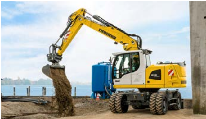
The A 918 Compact Litronic in use for earthmoving work in Kressbronn at Lake Constance (Germany)
