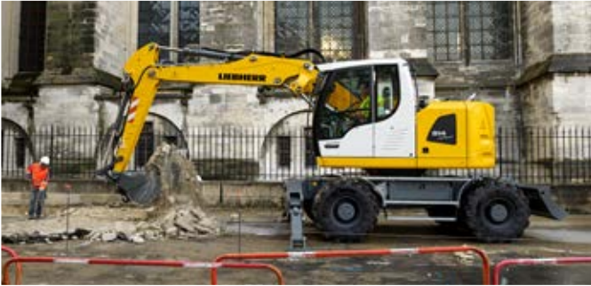
The A 914 Compact Litronic in use for road construction work in Reims (France)
