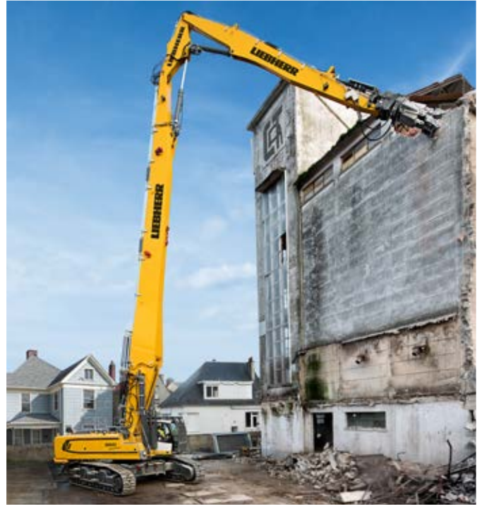
The crawler excavator R 960 used for the demolition of a silo in Frévent (France)
