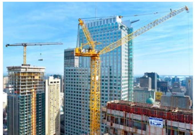
HC-L and EC-B cranes for the construction of a skyscraper in Canada
