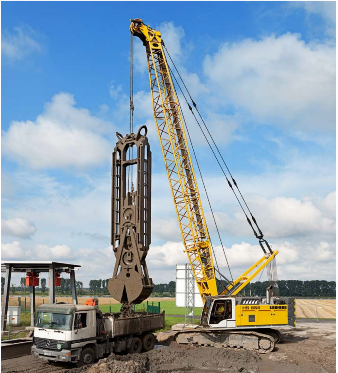
A duty cycle crawler crane from Liebherr at work with a slurry wall grab
